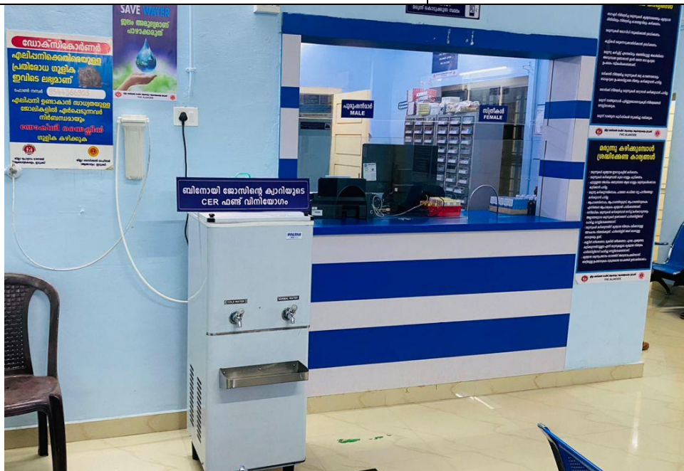
Figure 9: Photograph of Water Purifier Installed at PHC, Alakode
